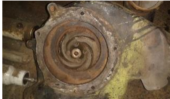
Figure 2: View from the pump's upper cover
